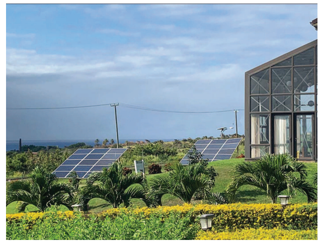
Solar PV Installations
