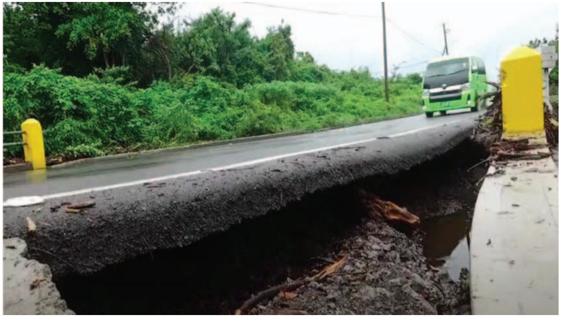
Area of washed out roadside on Nevis due to heavy rains associated with the passage of Hurricane Tammy in October 2023
