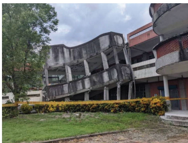
Damage to Chunri Elementary School in Hualien County. Photo credit: CNA.
