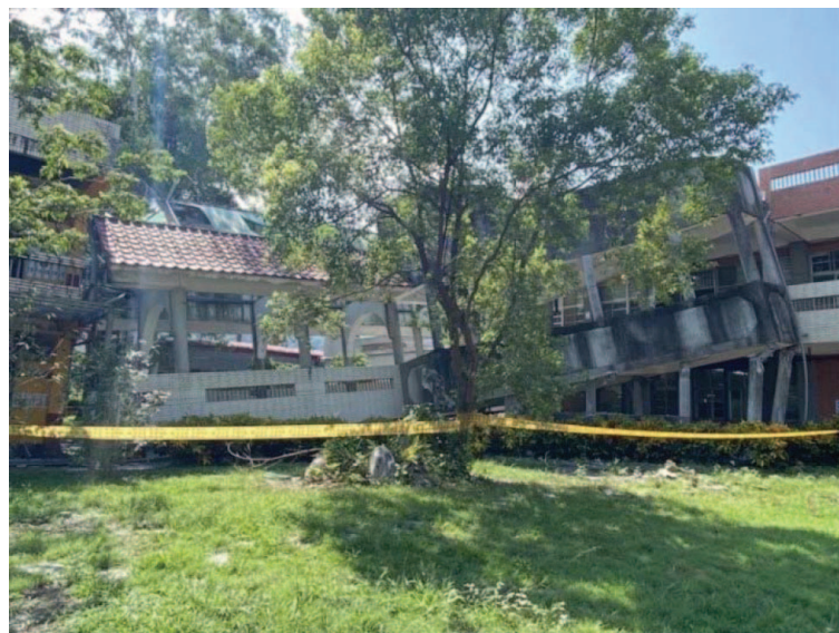
Damage to Chunri Elementary School. Photo credit: MOE.
