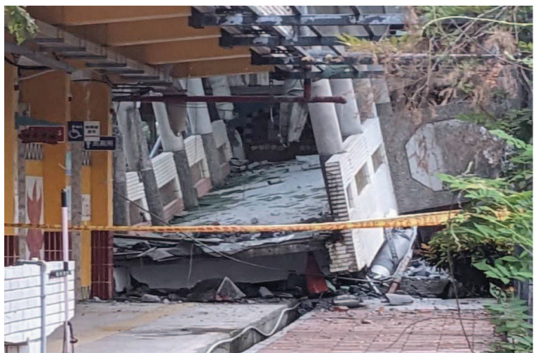
Damage to Chunri Elementary School in Hualien County. Photo credit: CNA.
